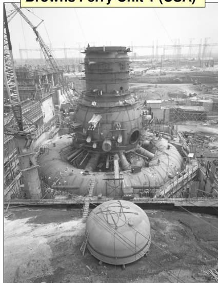
Browns Ferry Unit 1 drywell and wetwell under construction. (a BWR/4 using the Mark I containment)
